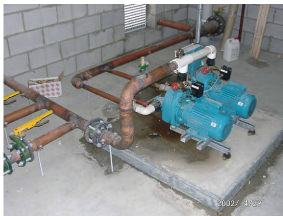
Figure 7. Water supply pumps above penthouse suite
