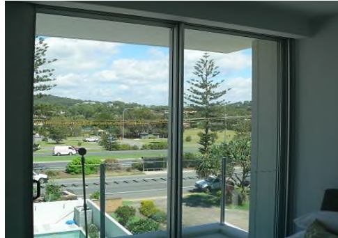
Figure 5. Acoustic double glazing system to manage aircraft noise.
